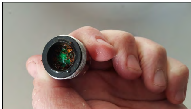
Picture of an aerator with particulate
